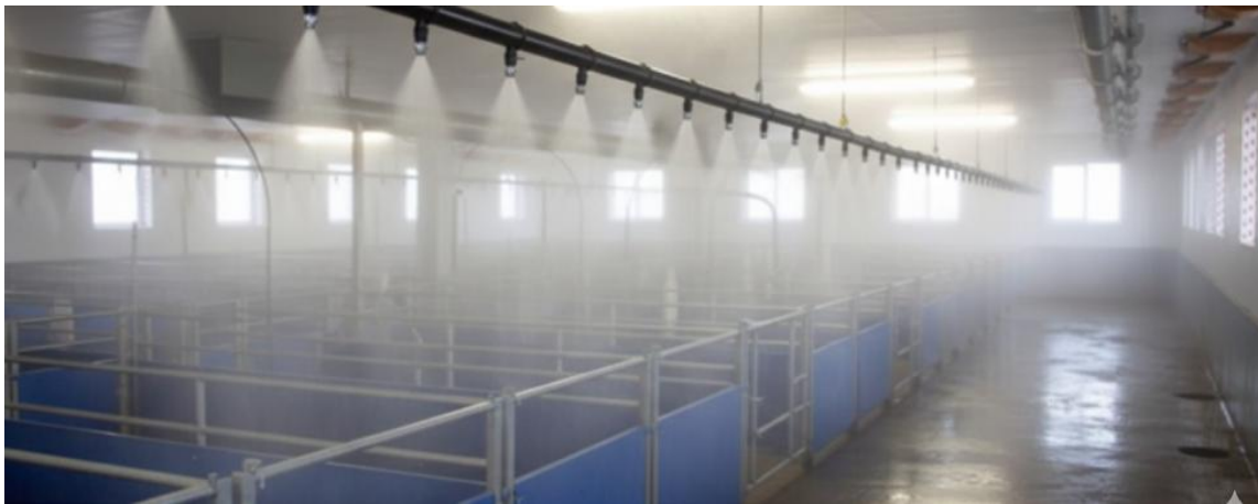
Fig. 2. Cooling system manufactured by LUBING
