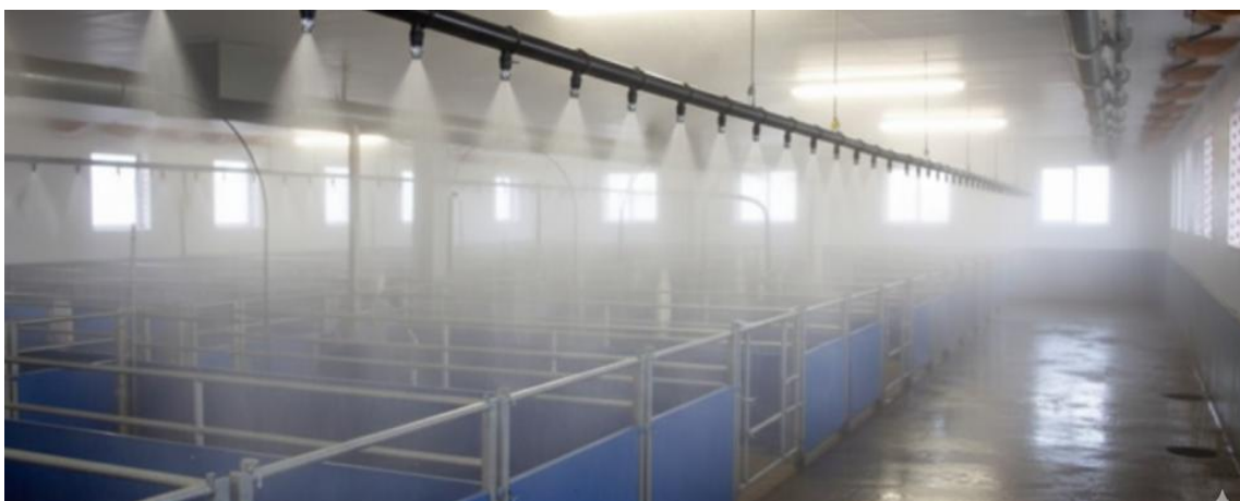
Fig. 2. Cooling system manufactured by LUBING
